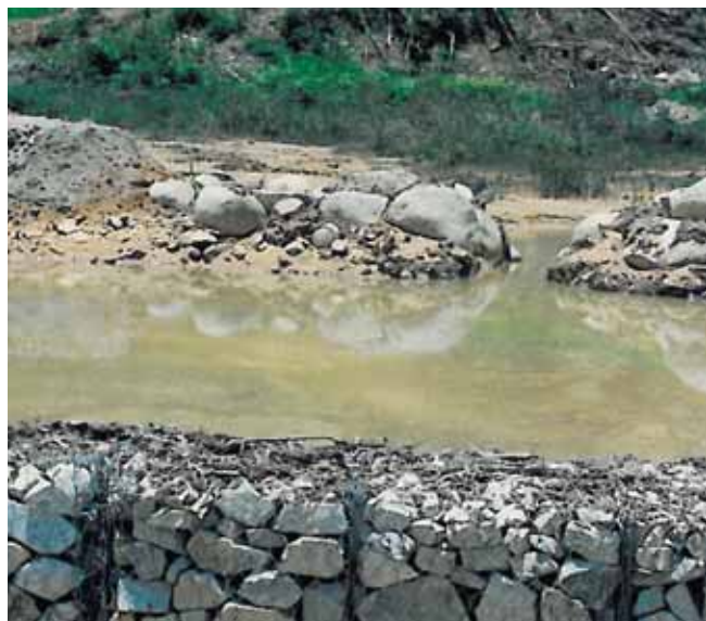
Silt trap and rip-rap measures adopted for river protection at Perak for the Electrified Double Track Project (Ipo-Padang Besar).
