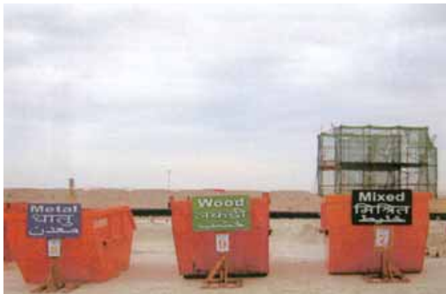
Proper waste management is implemented at New Doha International Airport (NDIA) and other project sites.
