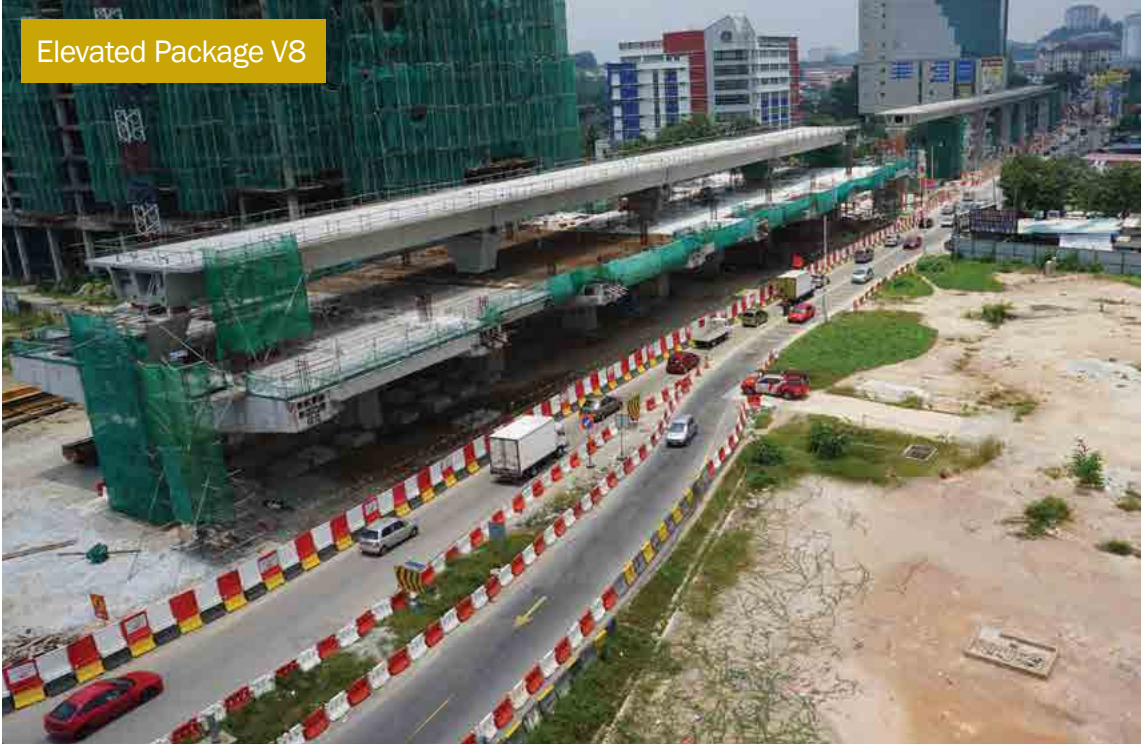
Construction works for concourse level in progress at the future Sungai Kantan MRT Park n Ride Station at Jalan Cheras-Kajang (near KPJ Kajang Hospital).
