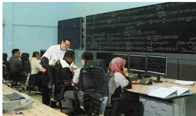
Picture shows the completed northern Centralised Traffic Control (CTC) located in Bukit Mertajam, Penang. It controls the railway signalling that centralised the train operations according to the railway system designated along the northern Electrified Double Track Project (Ipoh – Padang Besar).
