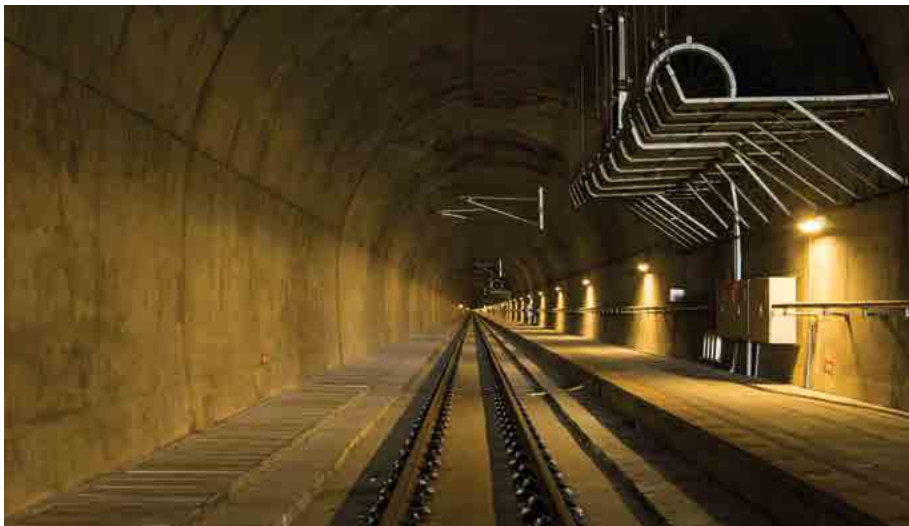
Interior of the 3.4km twin-bore tunnel in Bukit Berapit, Perak. The tunnel is completed with the installation of overhead electrification wiring and tracks.
