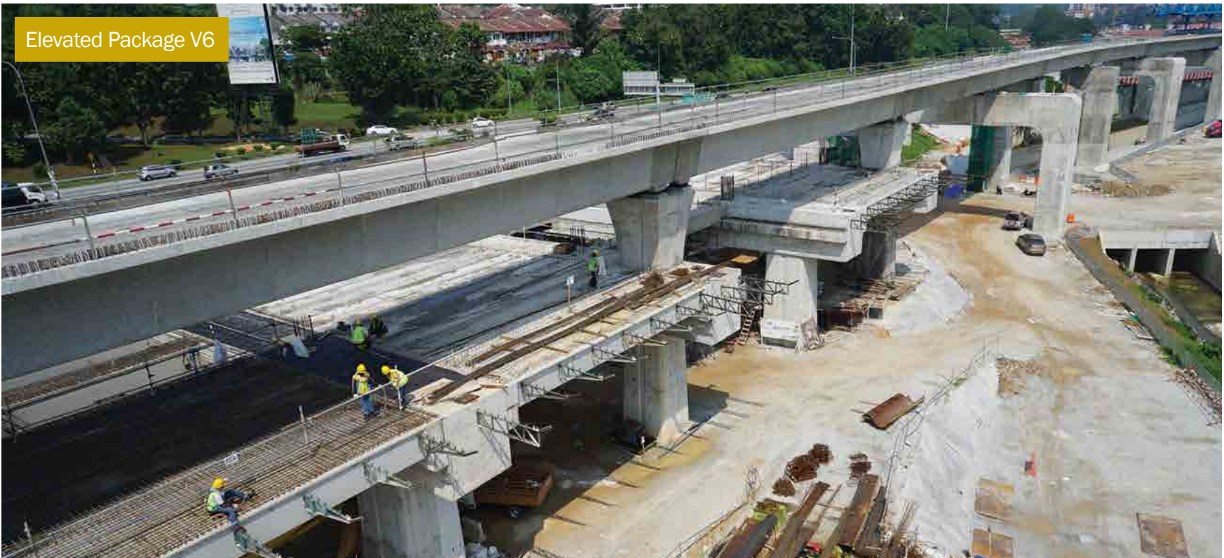
Six out of eight spans were completed for the concourse level of the future Taman Suntex MRT Station, along the Cheras-Kajang (Grand Saga) Highway.
