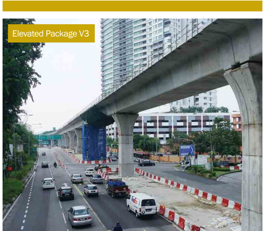
Parapet installation in progress for the completed MRT guideway along Jalan Damansara, passing Sinaran TTDI condominium at TTDI as the alignment heads towards TTDI MRT Station.
