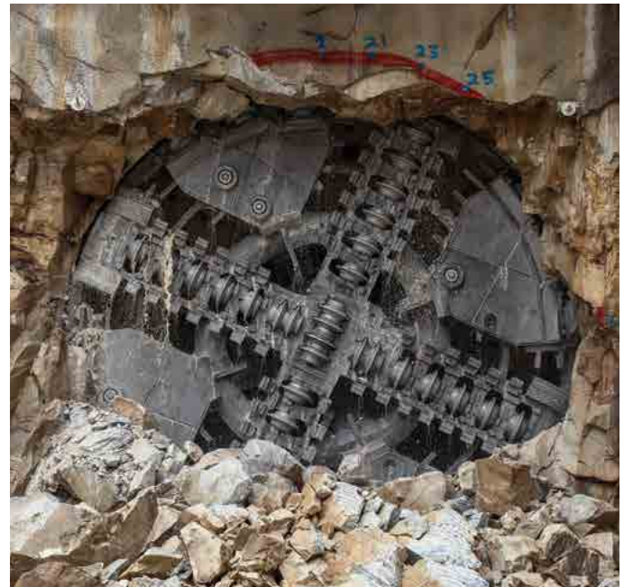
Breakthrough of the first VD TBM at Tun Razak Exchange (TRX) MRT station.
