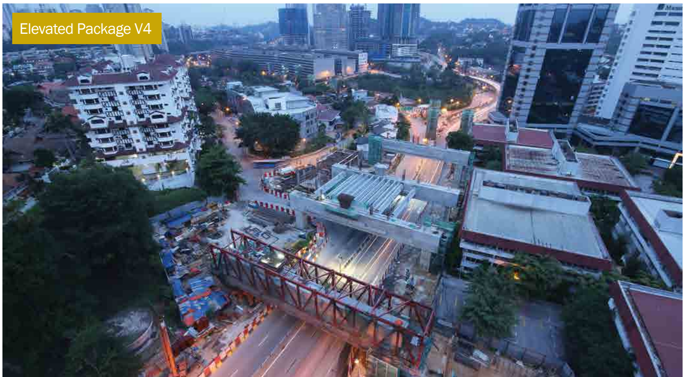
Beam launching and portal rebar works in progress for the future Semantan MRT Station, located along Jalan Semantan. Comprehensive traffic management plan was implemented to accommodate construction works amidst heavy traffic.
