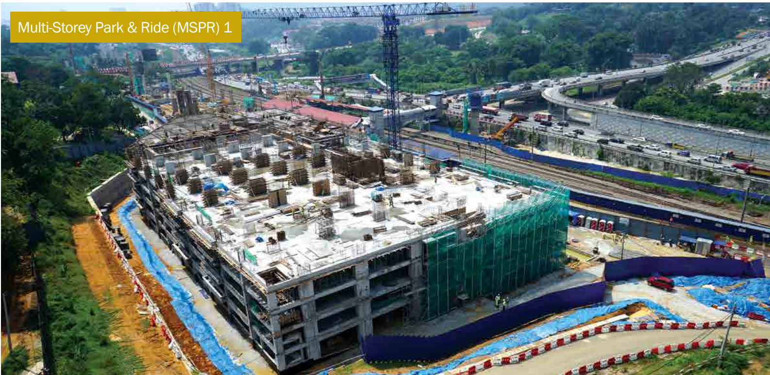
Advanced construction of the multi-storey park-and-ride building for the Sungai Buloh MRT Station which will integrate with KTM Komuter Sungai Buloh Station. The parking facility is expected to be completed within the second quarter of 2015.
