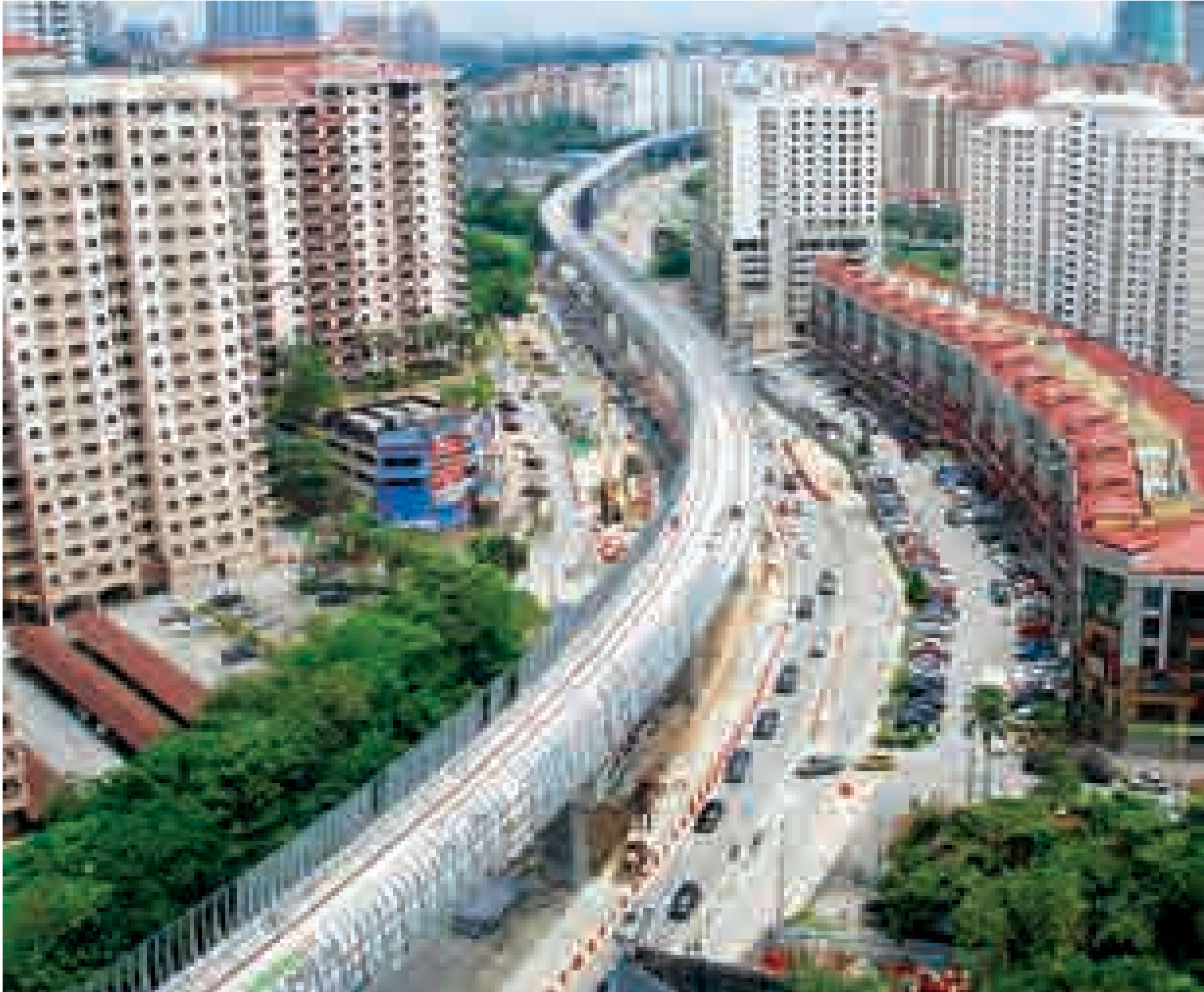
Viaduct noise barrier installation in progress along Persiaran Surian, next to Pelangi Damansara condominium.
