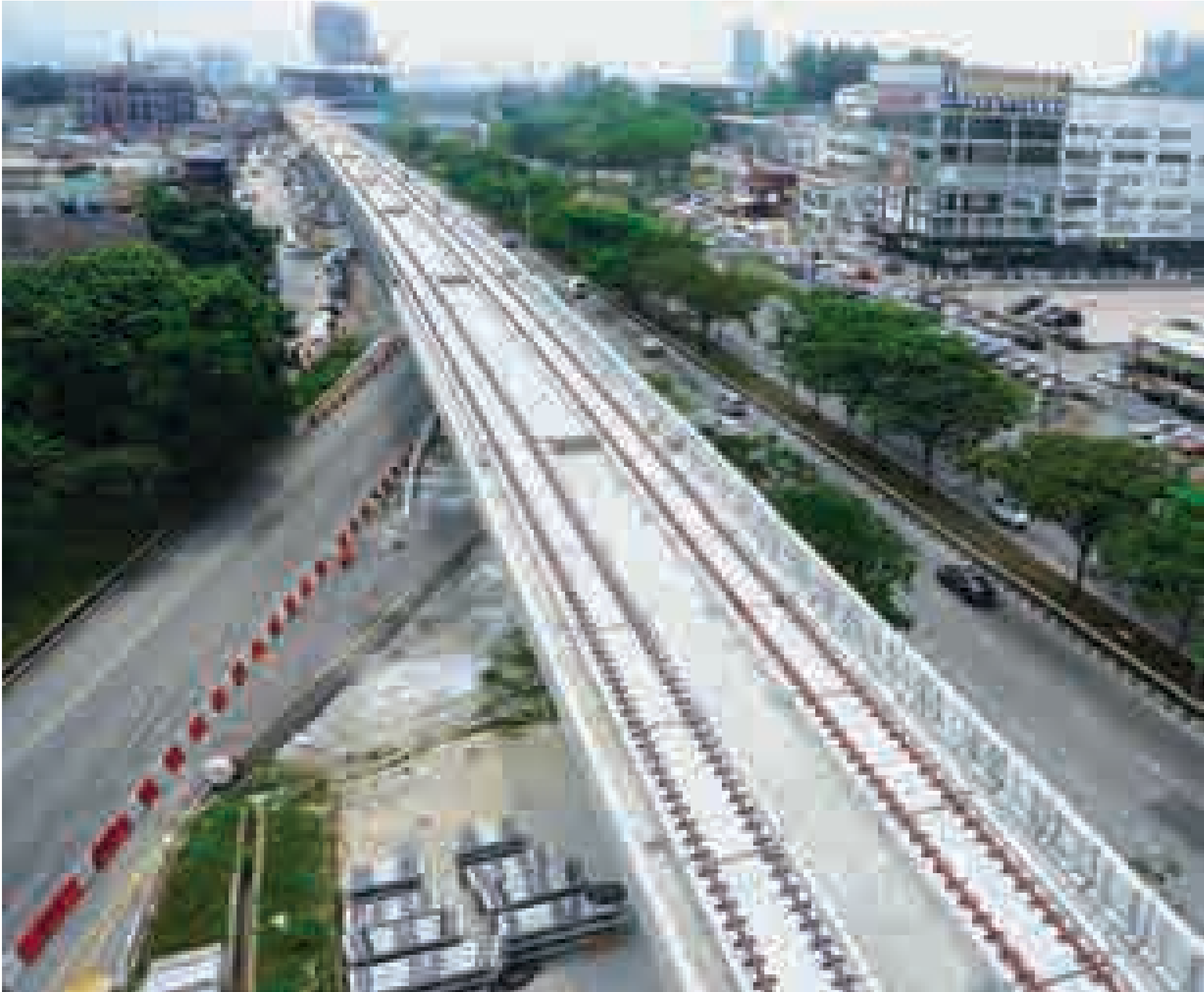
Ongoing track works on viaduct along Jalan Cheras, heading towards the Taman Midah Station.
