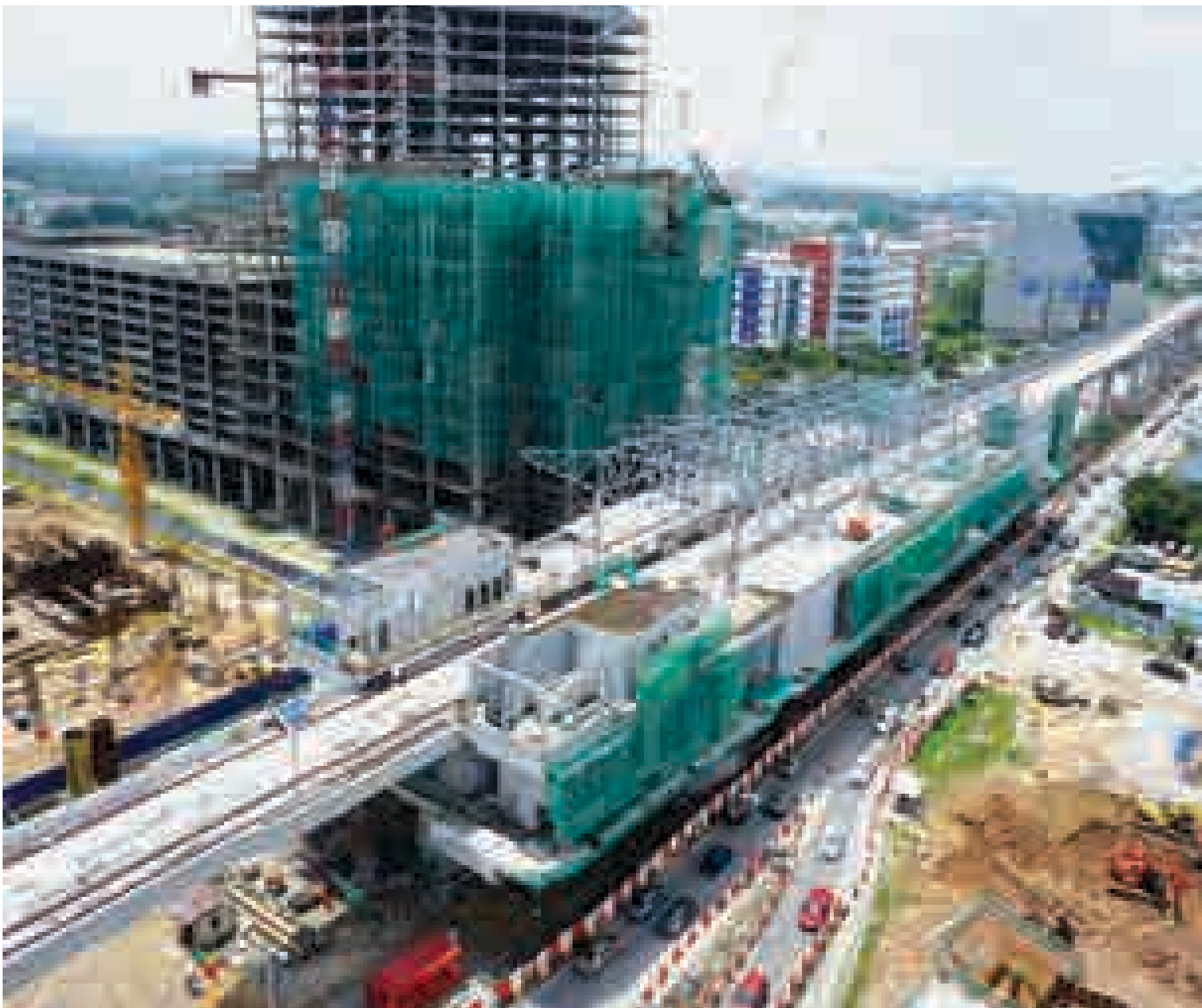
Roof truss installation, architectural and M&E works are concurrently taking place at the Sungai Jernih Station. This station has two Multi Storey Park N' Ride (MSPR) buildings, with each located at both sides of Jalan Cheras.
