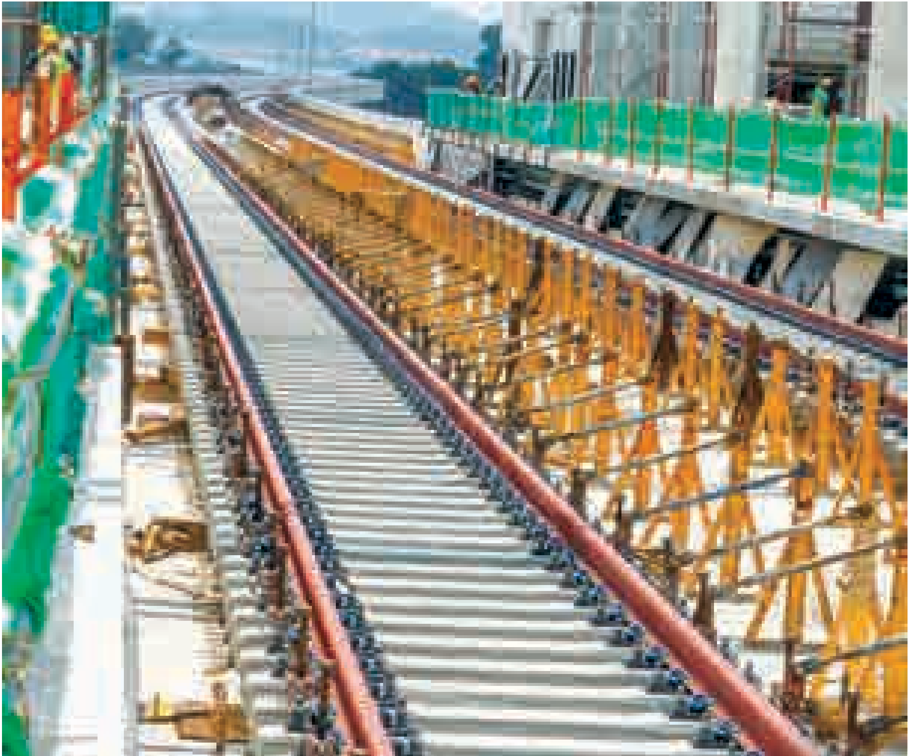
Systems, testing and commissioning, and trial run on the new rail tracks will take place for a period of six months, ahead of commencement of operations by mid-2017.
