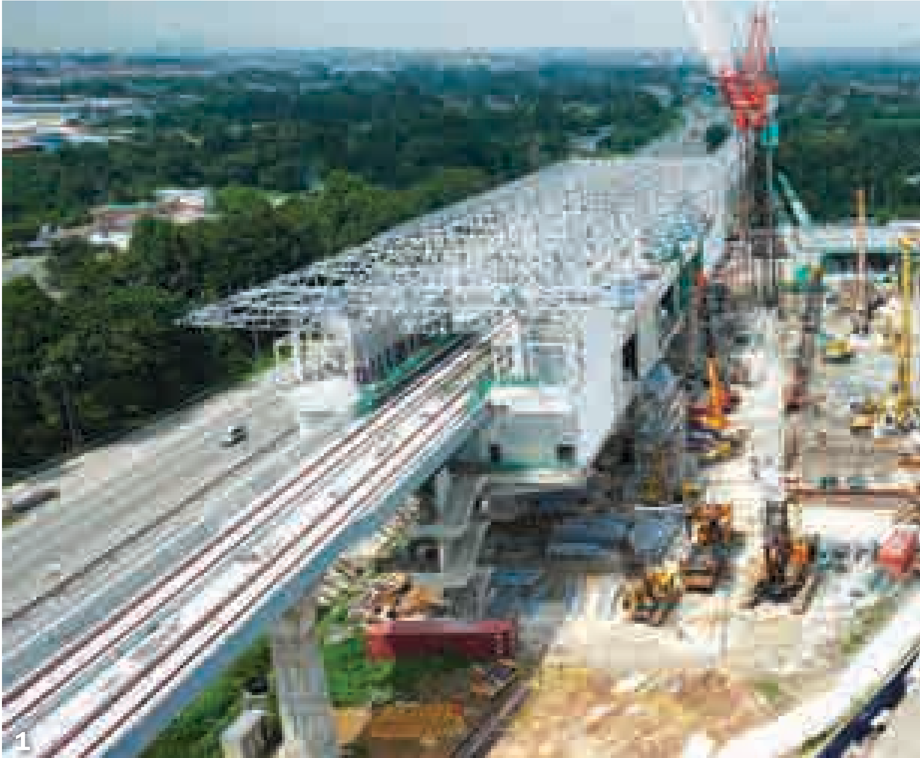
1, 2 and 3: Ongoing roof truss installation, architectural and M&E works at the Bukit Dukung Station are near completion.
