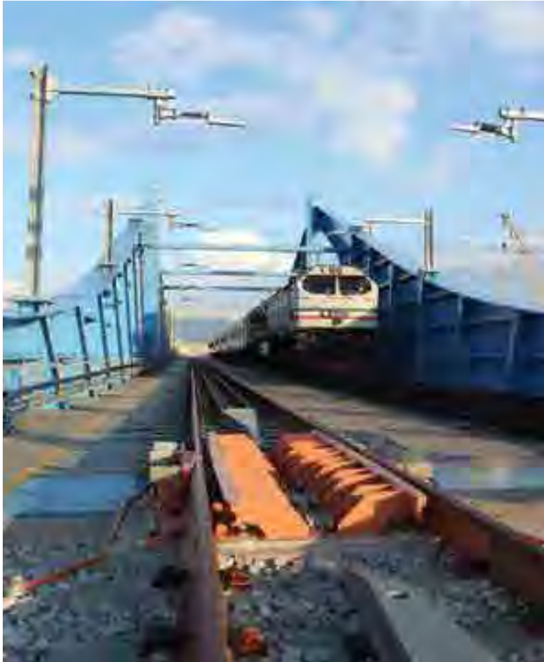
The newly completed 282m Prai Swing Bridge, Penang, is taking over the existing 50-year-old single-track railway bridge which was built in 1960s. This swing bridge will be electrohydraulic driven, with a 90m-mid span which is able to rotate and swing.
