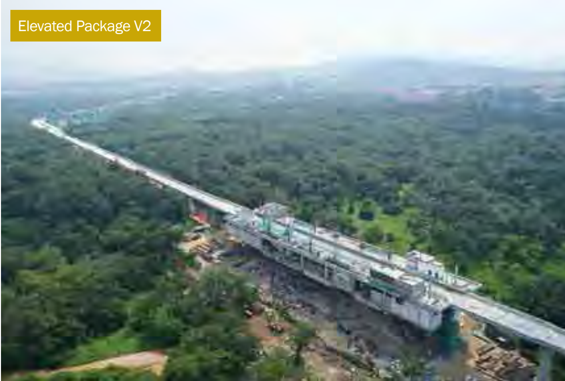
Advanced stage of concreting and formworks for the future Kwasa Sentral MRT Station in the former Rubber Research Institute area.
