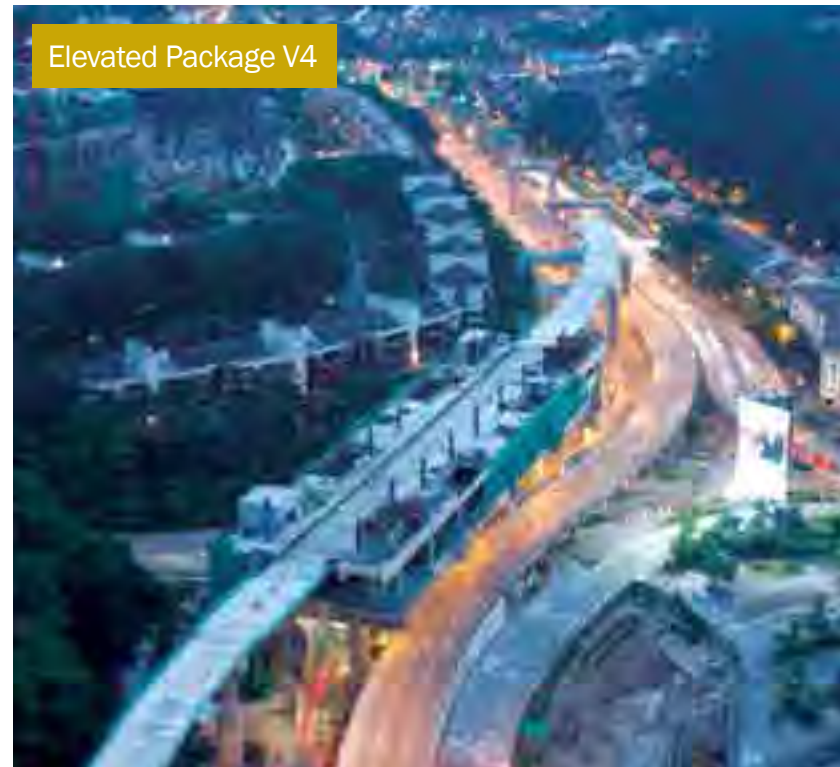
Concreting and formworks for the future Pusat Bandar Damansara (PBD) MRT Park n Ride Station in progress, at the busy intersection of Ma'arof Interchange along SPRINT Highway.
