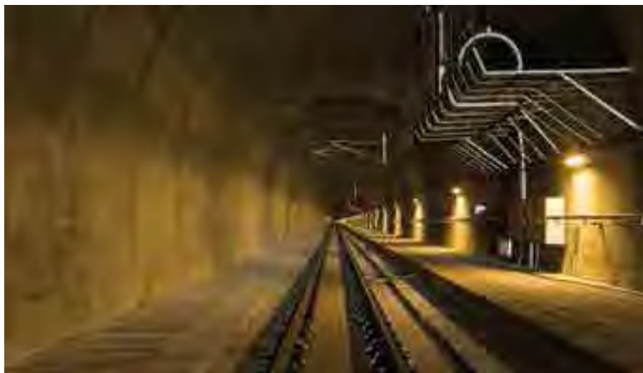
Interior of the 3.4km twin-bore tunnel in Bukit Berapit, Perak. The tunnel is completed with the installation of overhead electrification wiring and tracks.
