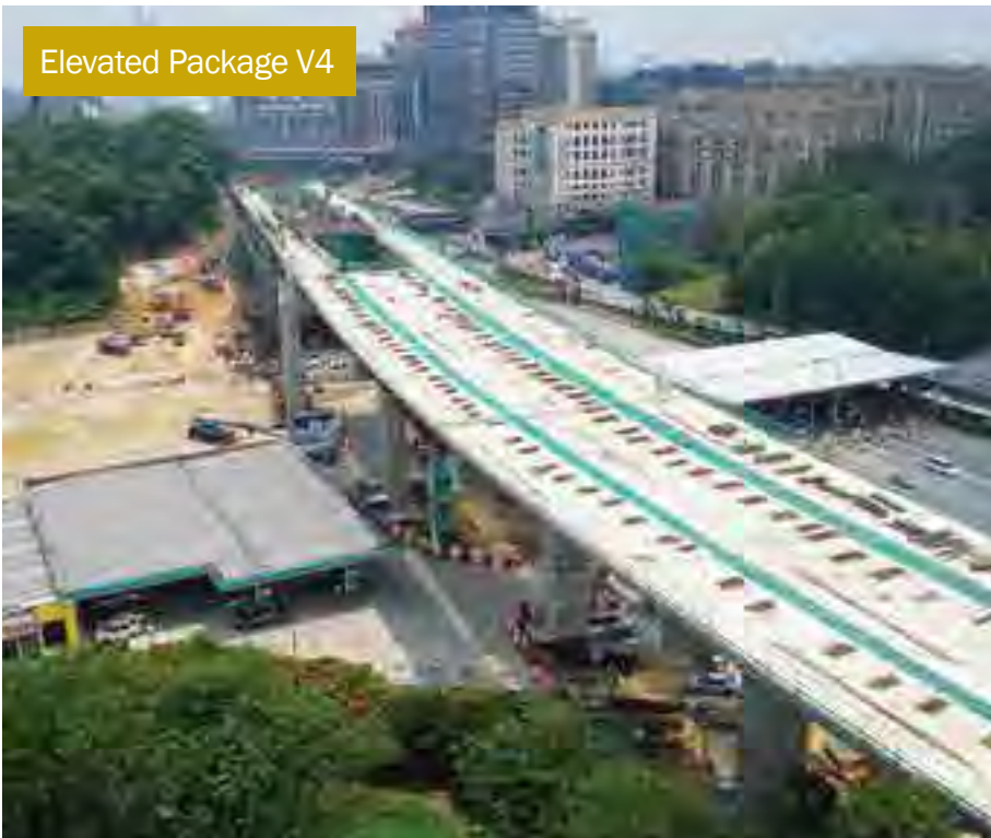
Construction of the station's concourse and platform levels is fast progressing for Phileo Damansara MRT Station at Section 16, along SPRINT Highway.
