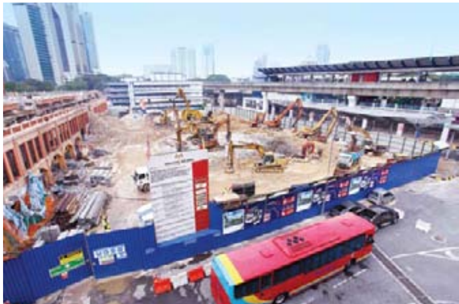
Demolition works at the Pasar Seni KVMRT station site was completed in September 2012. This future underground station will be integrated with the existing Pasar Seni LRT station
