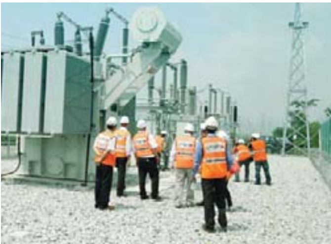
A total of nine feeder stations will transform raw 132kv electricity tapped from the local TNB power grid into 25kv to power the trains' movements. The first completed and energised feeder station is pictured here at Lahat, Perak
