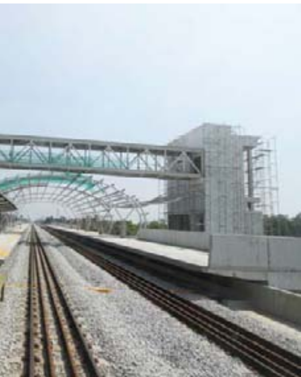
All new KTMB stations along the new double track are designed with a modern exterior and will be equipped with the latest station amenities for commuters' convenience. The picture shows the Bagan Serai KTMB station that has achieved substantial completion
