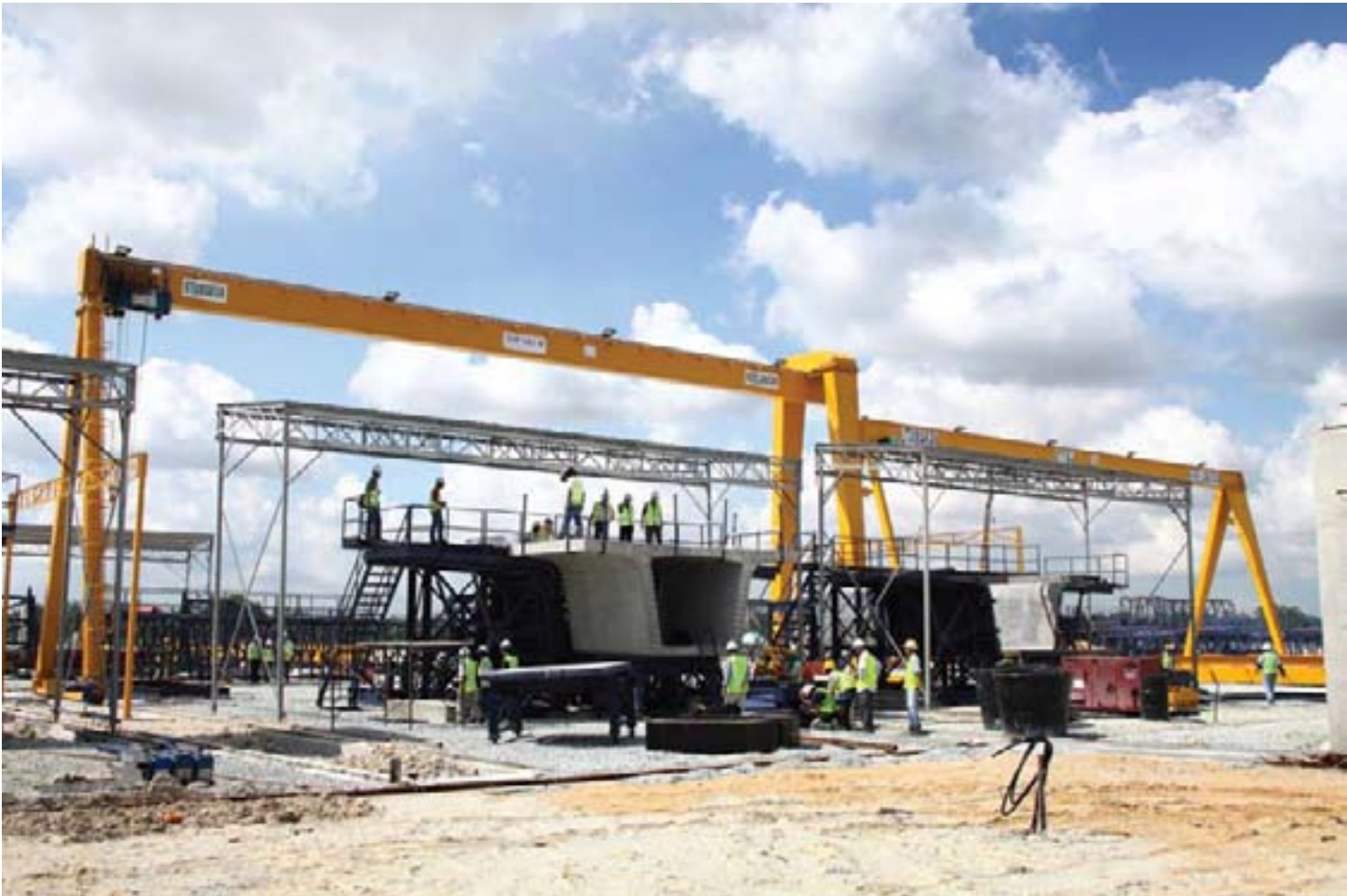
The Segmental Box Girder (SBG) Casting Yard in Sepang will be able to produce a total of 17,000 SBGs for the construction of the KVMRT's twin track. Each of these 11metres-wide SBGs weighs about 45 tonnes. The first delivery of SBGs is expected in January 2013, to be used for the V5 KVMRT package (from Taman Bukit Ria to Plaza Phoenix, Cheras)
