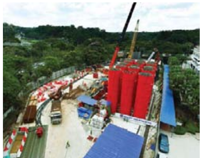
Diaphragm wall construction equipment have been installed and ready to commence works at the KL Sentral KVMRT station site
