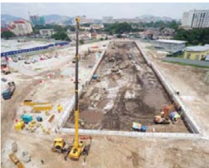
Construction works in progress in preparation for the Cochrane KVMRT station box, which will be integrated with the major redevelopment of Cochrane
