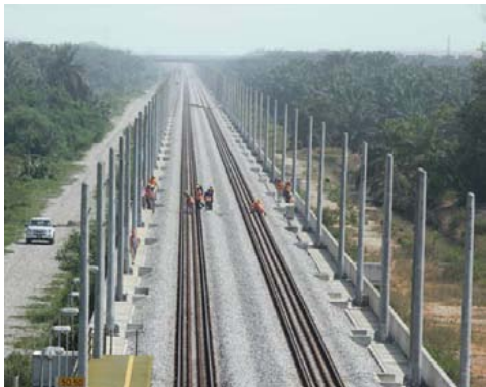
All infrastructure and track works, as well as Overhead Catenary System mast installation along the tracks leading to the Bagan Serai KTMB station have been completed
