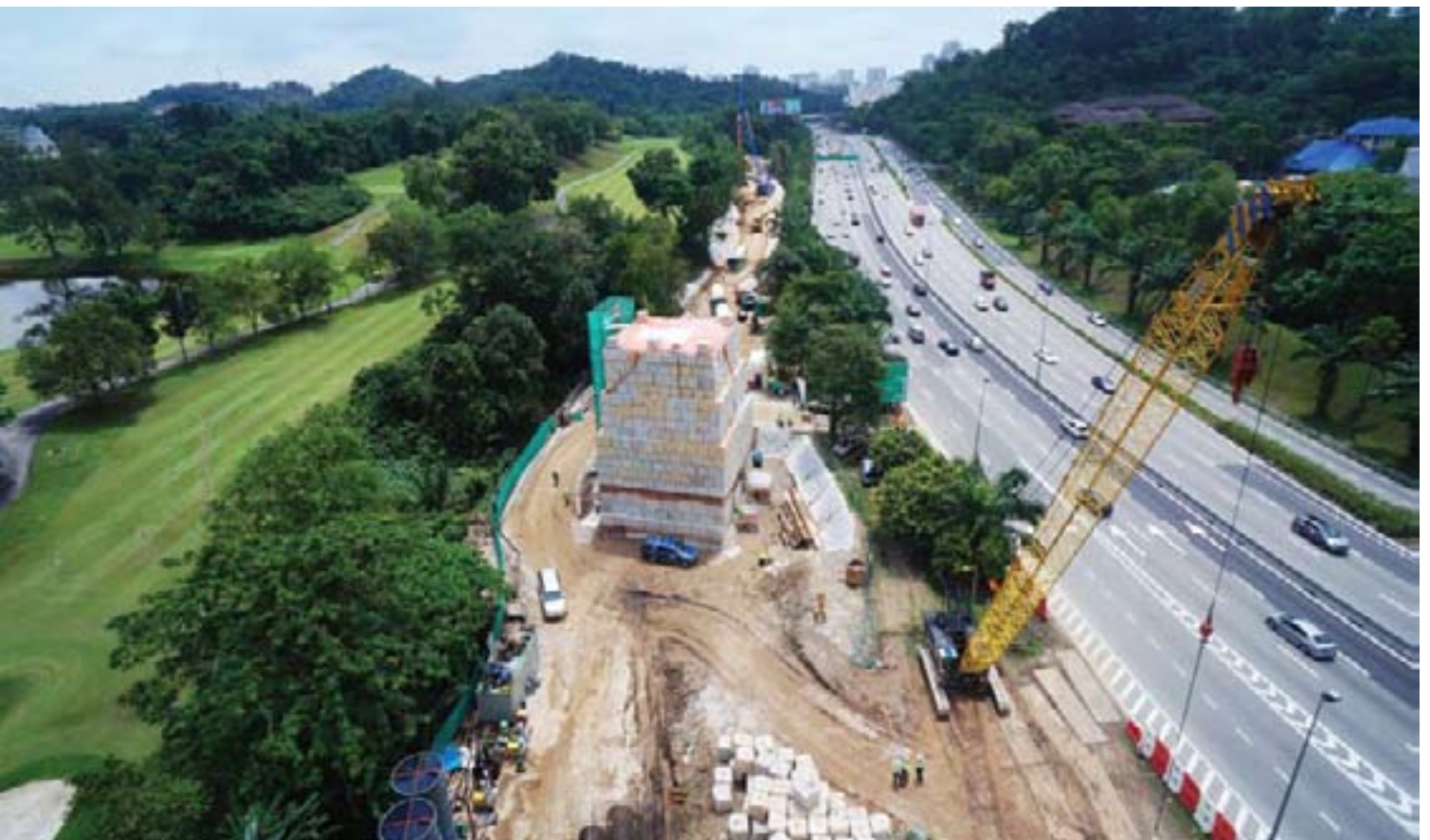
Construction for the KVMRT viaduct guideway and other associated works in progress, located next to the Malaysia Civil Service Golf Club (commonly known as Kelab Golf Perkhidmatan Awam, KGPA) alongside the Western Kuala Lumpur Traffic Dispersion Scheme (SPRINT) Highway
