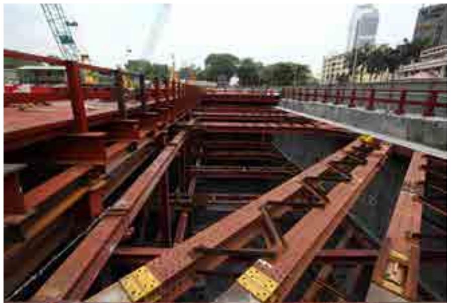
Excavation works has reached the third layer, while extensive strutting is still ongoing for the second layer of the station box at the Merdeka MRT station.
