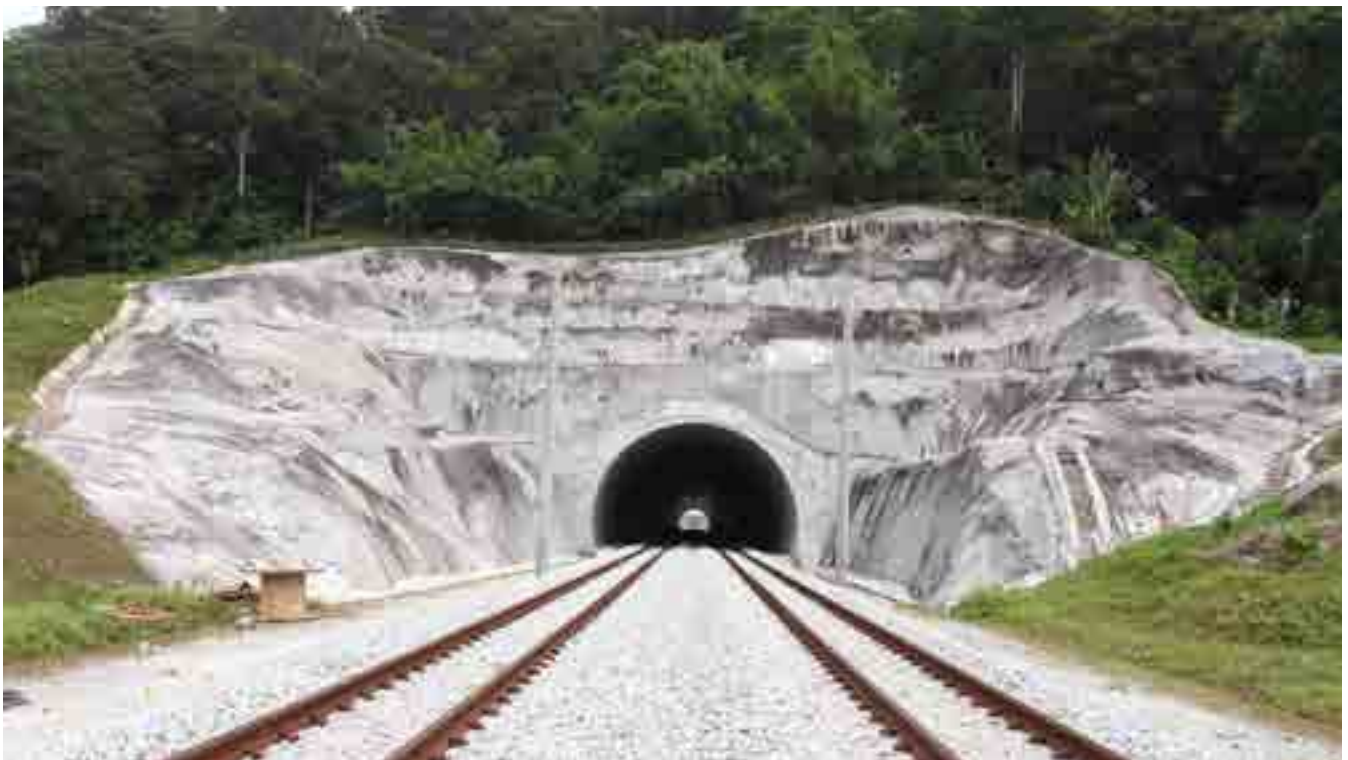
The fully completed Larut Tunnel at Bukit Larut, Perak, is the first railway tunnel built for electrified trains in Malaysia. The tunnel was commissioned in April 2013.
