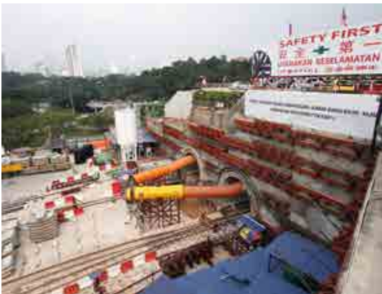
To support the fast-paced Kenny Hill formation tunnelling at the Semantan Portal, fresh air needs to be channelled into the tunnels 24/7 via ventilation ducts, while tunnel ring segments are systematically stacked waiting to be transported into the tunnels for installation.
