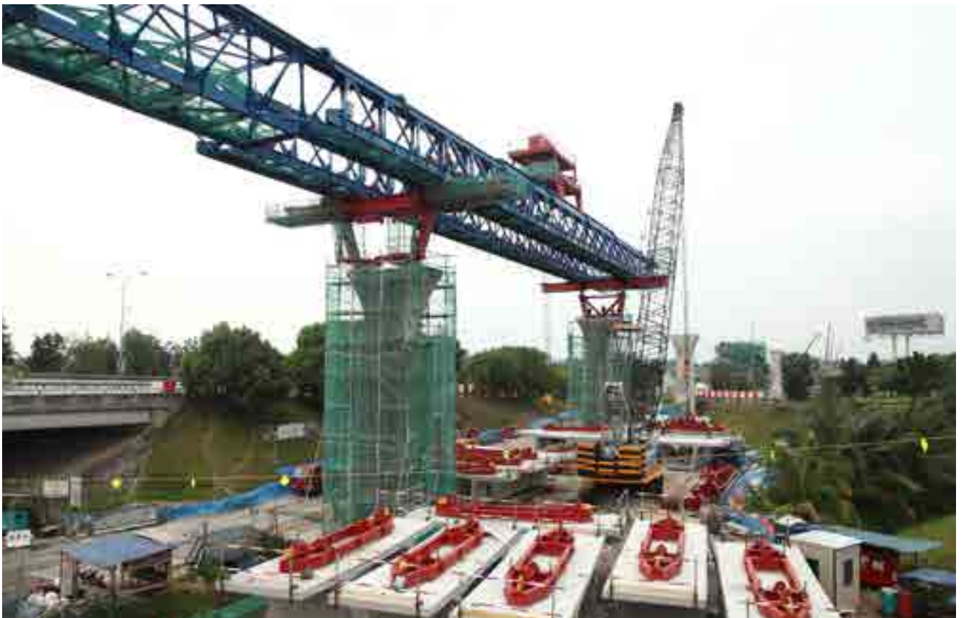
Viaduct construction is actively ongoing along the Grand Saga Highway for elevated viaduct package V7, where Launching Gantry (in blue) is used to lift, align and fix Segmental Box Girders (SBGs) (in white-coloured concrete) in place to form the permanent viaduct for the Sungai Buloh – Kajang Line. Each SBG weighs up to 50 tonnes.
