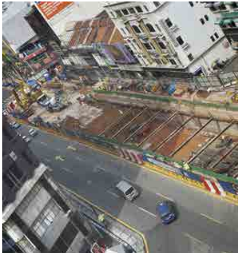
Extensive strutting works were completed to support excavation works at Bukit Bintang MRT station. With the floor mat for first panel of roof slab laid, next would be rebar fixing, followed by scheduled casting.
