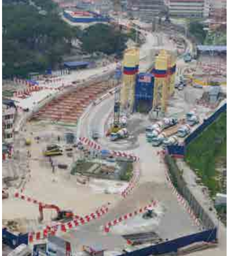
Picture shows the Maluri Portal, where the two VD TBMs from Cochrane will end its journey. Strutting to support excavation of the shaft (left), which forms part of the underground-elevated transition structure, was installed.
