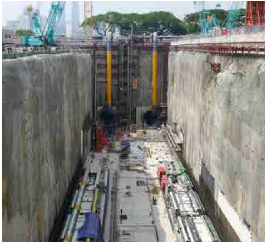
Assembly of the third and fourth VD TBMs in progress at the Cochrane Launch Shaft (foreground). These two VD TBMs will mine towards the Maluri MRT station. In the background are two tunnel mouths from which the first and second VD TBMs were launched earlier this year.
