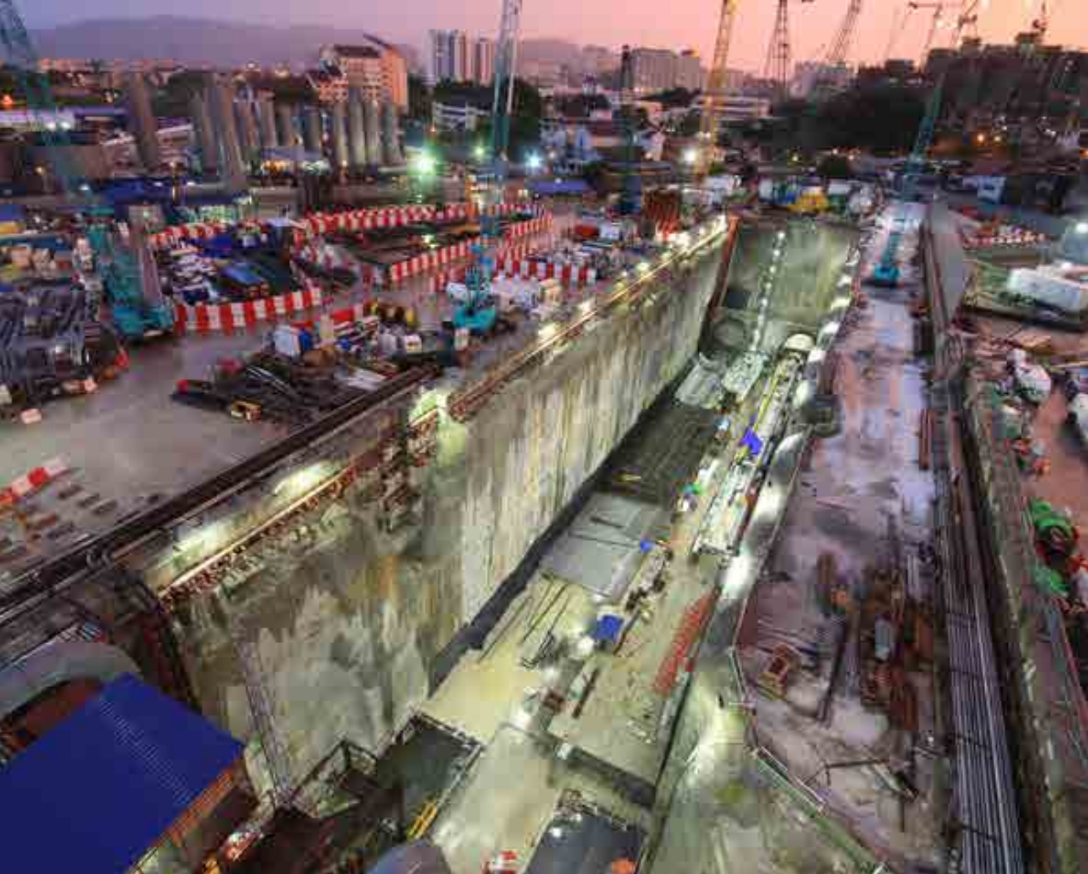
An aerial view of the Cochrane work site at dusk showing an almost fully assembled third Variable Density Tunnel Boring Machine in the Cochrane Launch Shaft that will tunnel towards the Maluri MRT station.
