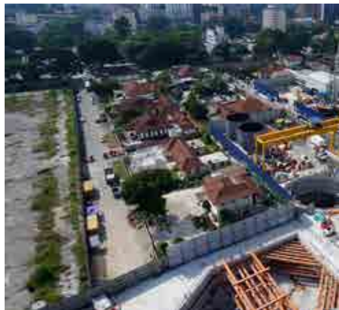
Strutting and heavy excavation for station box are well advanced at the Pasar Rakyat MRT station. Also seen in the picture (background) is the Upper Inai Launch Shaft, where one unit of VD TBM will tunnel towards the Bukit Bintang MRT station.
