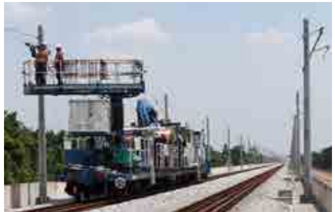
Ongoing installation of overhead electrification wiring along the Land Viaduct at Simpang Lima in Perak.
