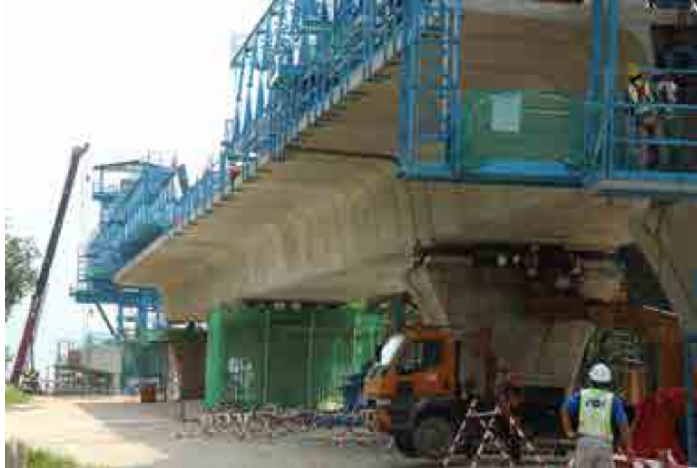
Erection of Launching Gantry between Pier KD 24 and Pier KD 25 and installation of Segmental Box Girders (SBGs) to form the elevated viaduct from Pier KD 26 till Pier KD 30 were progressing concurrently in elevated package V2 of the SBK Line.
