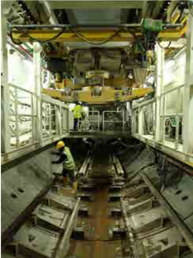
Workers are working hard to sustain the tunnelling momentum by installing temporary rail tracks (at the centre of the picture) to facilitate the transfer of tunnel ring segments into and excavated materials out from the tunnel at the Semantan Portal.
