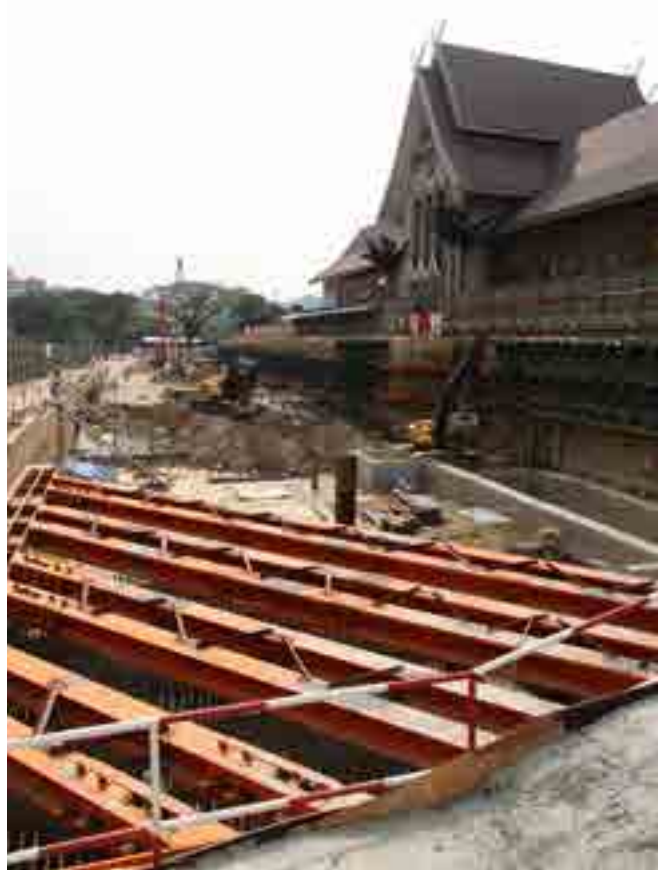
To safeguard the continuous integrity of the National Museum building, located just next to the KL Sentral MRT station work site, extensive monitoring of ground movements caused by construction works was carried out.
