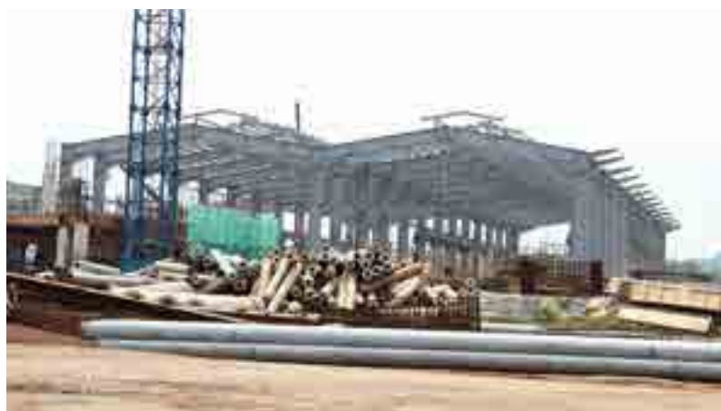
Erection of steel frame for the building that will house the SBK Line's rolling stock for regular upkeep and maintenance is ongoing at the Sungai Buloh depot.
