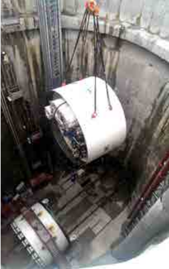
VD TBM assembly at the 30m-deep Upper Inai Launch Shaft. Picture shows the front shield of the VD TBM being lowered into the shaft during the assembly process.
