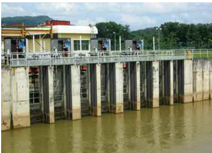
▲ Raw water intake at Rasa Treatment Plant
