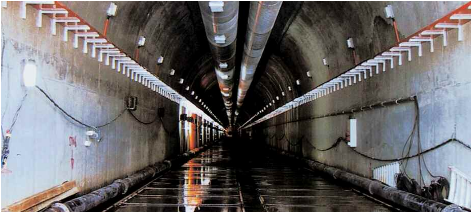
▼ SSP3's Dam Diversion Tunnel, which employed the controlled drilling and blasting method
