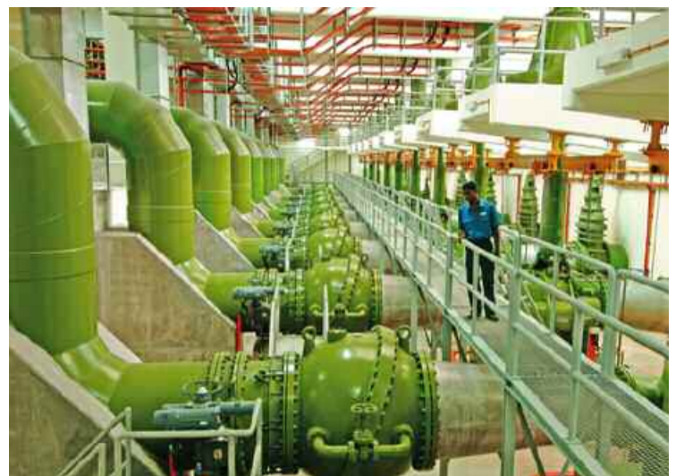
▲ Raw water pumps at Bukit Badong intake
