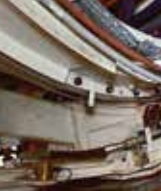
MRT2 (KUALUMPUR) Tunnelling activities for the country's second MRT Line have come to an end.
