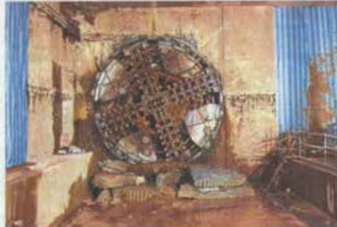
Level achieved: The cutter starting together cut through 17.7m below ground through underground of the future MRT PutraJaya Line at 17.7m. The cutter starts a total distance of 17.7m from the Station Centre (SC) station passing under Jalan Siman, Jalan Bangi, Jalan Ampang and under the MRT PutraJaya Line (PTJ) station to 17.7m.
