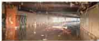
Inside SMART Tunnel after the dewatering process and before cleaning takes place.
